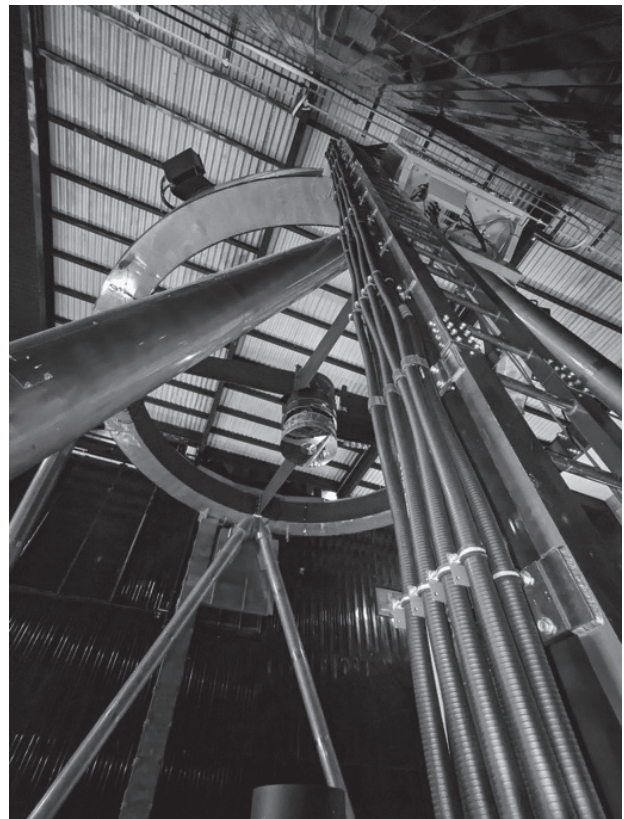
Figure 2: All 4 science fiber cables installed on the telescope, holding ~2400 optical fibers (May 2023).
